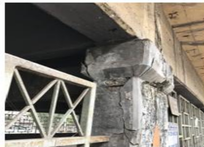
Figure 3. Structural cracks were seen on the columns
