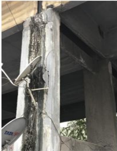
Figure 1:- Cracks in column number 6A due to satellite dishes.
