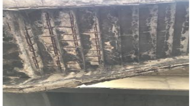
Figure 2. Exposed reinforcement on the underside of the staircase.
